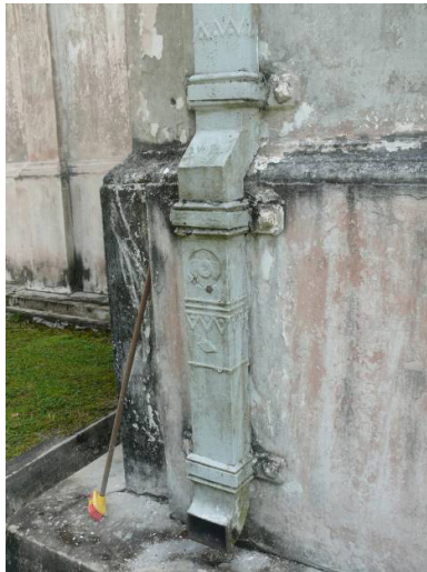
Photo 16: Inefficient water drainage due to improper water funnel design or damage inhibits water flow
