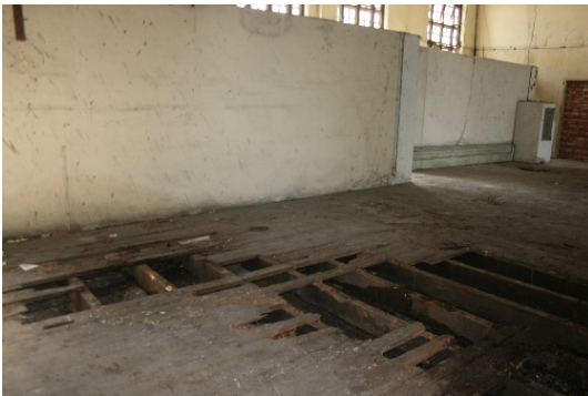
Photo 11: Damaged wood caused by termite attack and wood rot Source: Old Post Office Conservation Works Project, Ipoh, Perak, 2009
