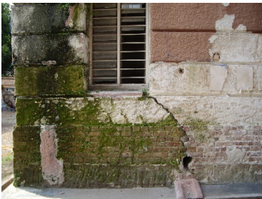
Photo 6: Moss and/or mould growth on wall surfaces Source: HSBC Building Conservation Project, Melaka, 2009
