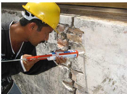
Photo 8: Conservation stapling works on the wall surface to strengthen the structure Source: Penghulu Natar House Conservation Project, Merlimau, Melaka, 2009
