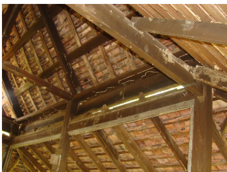
Photo 2: Termite attacks on the roof frame Source: Penghulu Natar House Rehabilitation Project, Merlimau, Melaka, 2009
