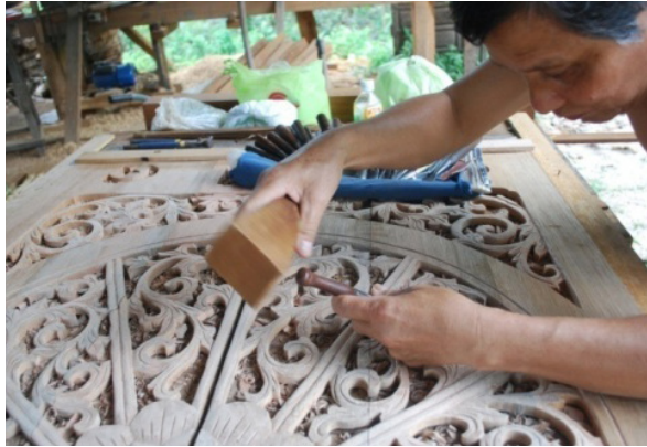
Photo 19: Carving wood filigree (kerawang) on a window panel Source: Ihsaniah Iskandariah Mosque Conservation Project, Kampung Kuala Dal, Perak, 2009
