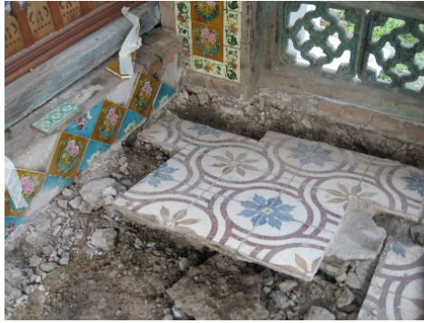
Photo 13: Conservation works on broken floor tiles Source: Penghulu Natar House Conservation Project, 2009
