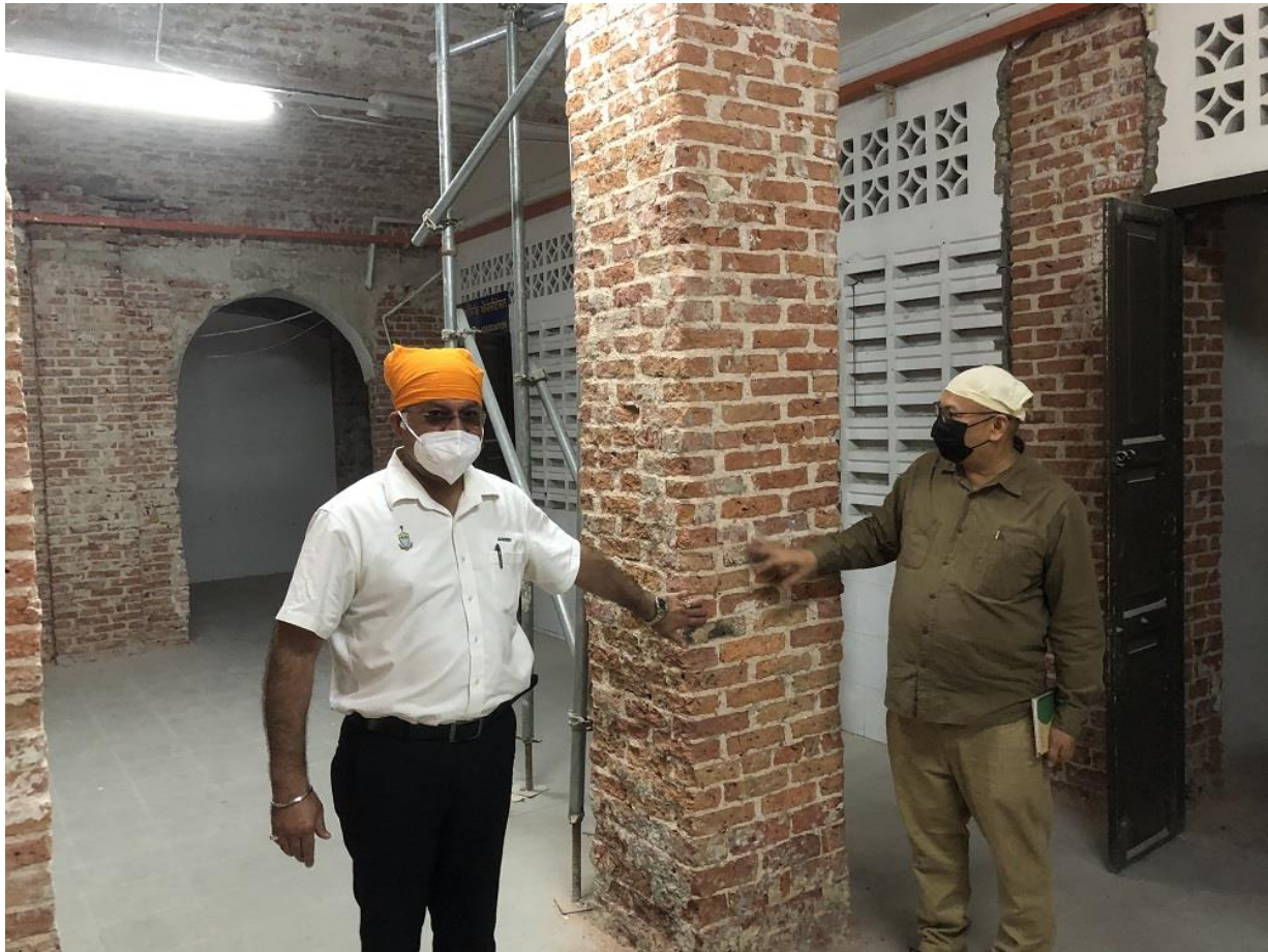
State exco Jagdeep Singh Deo and Penang heritage commissioner Rosli Nor (right) at the Wadda Gurdwara Sahib which is currently undergoing massive restoration works. — Picture by Opalyn Mok
